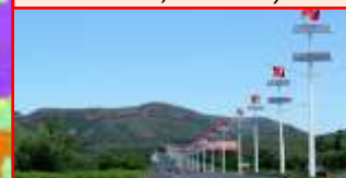
Solar Street Lighting, USA
