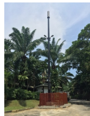
Foto : High Speed Broadband Tower
